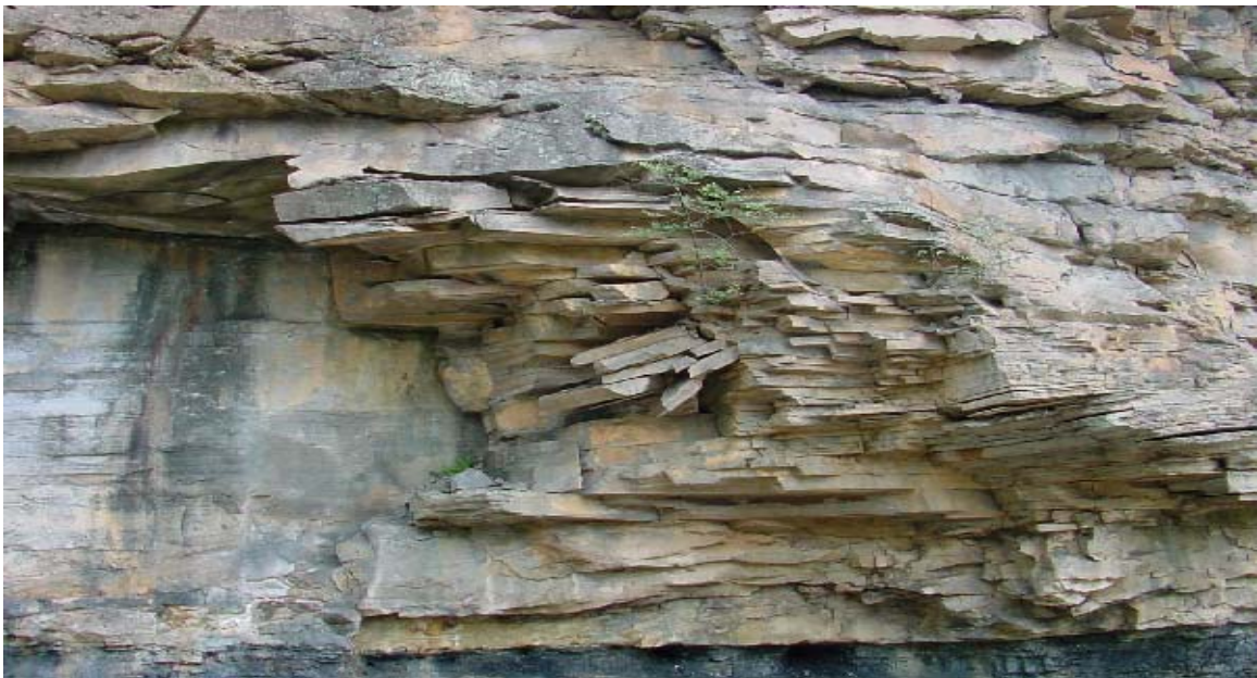
Figure 4: Structural discontinuities such as “joints, faults, bedding planes, or fissility” are the primary cause of rockfall
