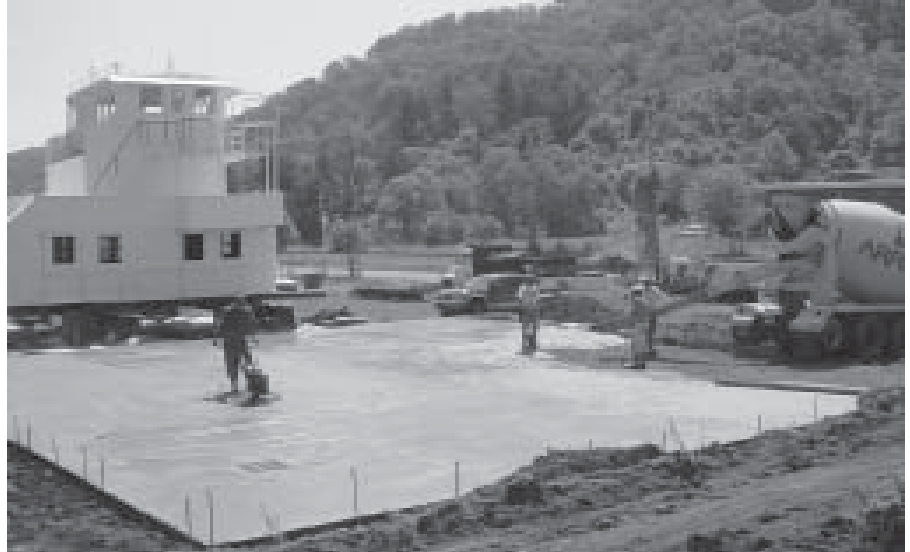
Above: RTI Research Associate John Ball, PE, designed and provided construction oversight in converting "The Warren" into a facility used to train professional, volunteer and maritime firefighters in Huntington, W.Va.
